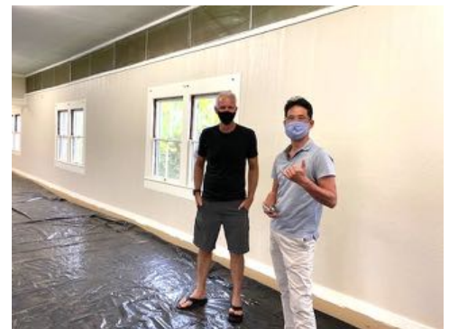
Shaun and Kai check on the painting of the social hall interior.
